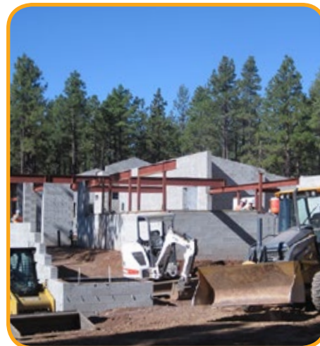
Construction on the new building is moving quickly with an expected completion date of Spring 2014.
